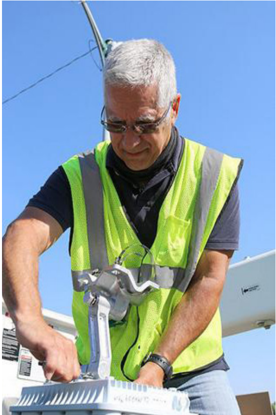
A bracket being mounted on a SmartWave AP. Source: Council Bluffs School District
